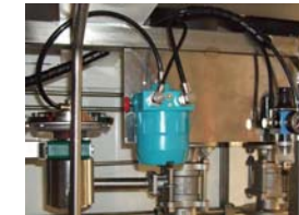
Pic. 3) Pressure Ramping regulators:
